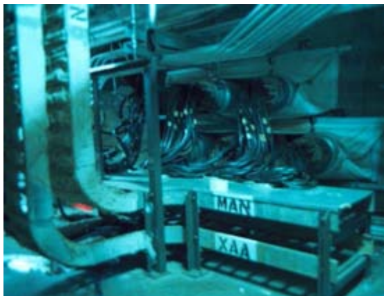
Power cables run through trays, conduits and tunnels, impeding the ability to inspect them, and to detect and suppress fires.
