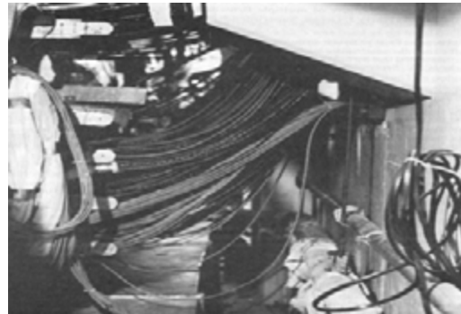
Hundreds of miles of electrical cables run through dozens of fire zones in a typical U.S. nuclear plant.
