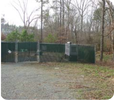
OWASA Pump Station
