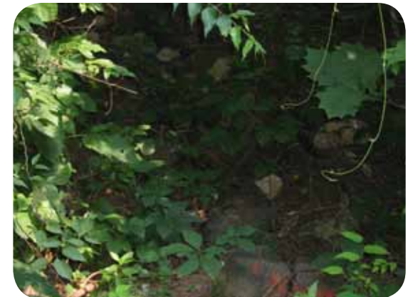
6 Major drainage problems along trail corridors should be addressed by staff or by an outside contractor when storm water issues become a hazard. Major drainageways such as this one should be maintained.
