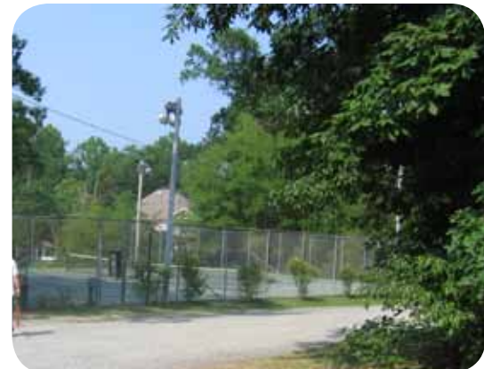
5 The tennis court needs new vinyl coated chain-link fencing. The vegetation along the perimeter of the tennis court needs to be removed. An ADA accessible route should be installed from the sidewalk to the tennis court.
