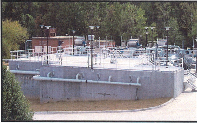
The new, enclosed “headworks” completed in July, 2007 to address a major odor source identified in a consultant’s odor study.
