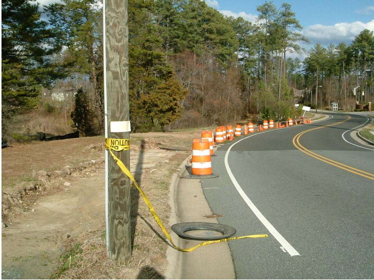
Photo 4a: The unfinished and deteriorating bus pull-in.
