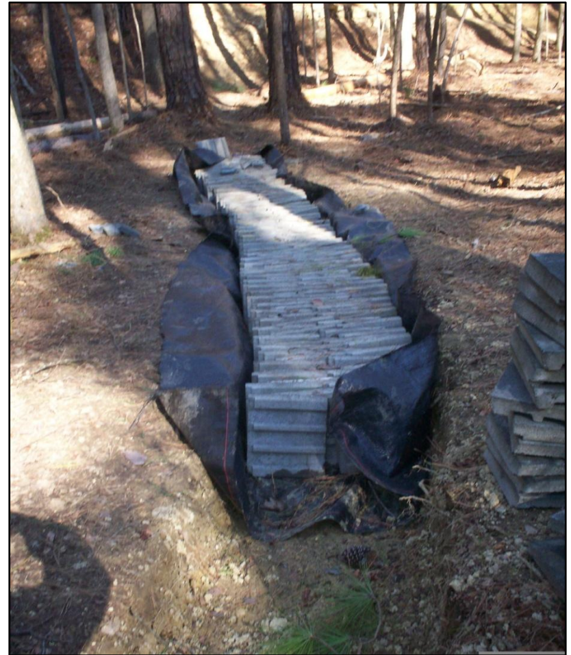
Roofing tiles from Venable Hall pitched to 'armor' a wet & muddy trail
