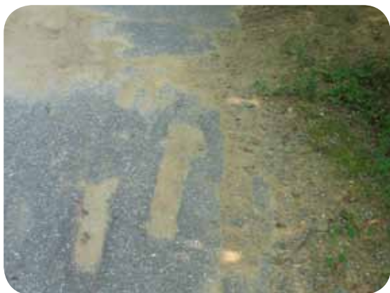
1 The length of the corridor has vegetation encroaching the edges of the trail's surface and causing the trail to crumble and crack. Sediment is also an issue due to clogged drainage pipes. The surface condition of the asphalt paving is fair, except for damaged areas such as the equipment damage shown above.
