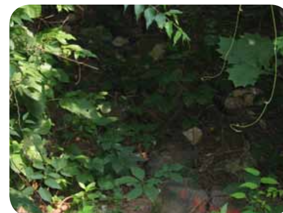
6 Major drainage problems along trail corridors should be addressed by staff or by an outside contractor when storm water issues become a hazard. Major drainageways such as this one should be maintained.
