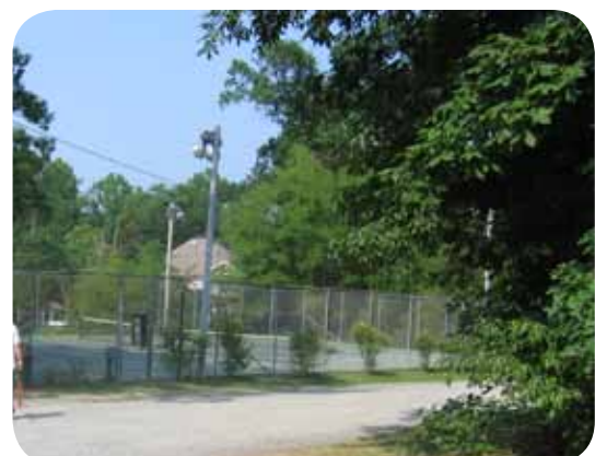
5 The tennis court needs new vinyl coated chain-link fencing. The vegetation along the perimeter of the tennis court needs to be removed. An ADA accessible route should be installed from the sidewalk to the tennis court.
