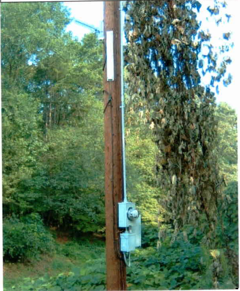
(B) Examples of ClearSKY radio enclosure, power meter and antennas on a Duke wooden power pole
