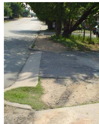
Rosemary Street, 13 Incomplete Sidewalk
