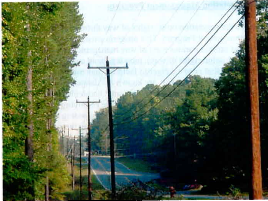
Three Phase Distribution Line
