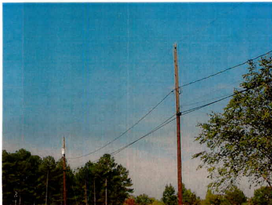
Single Phase Distribution Line
