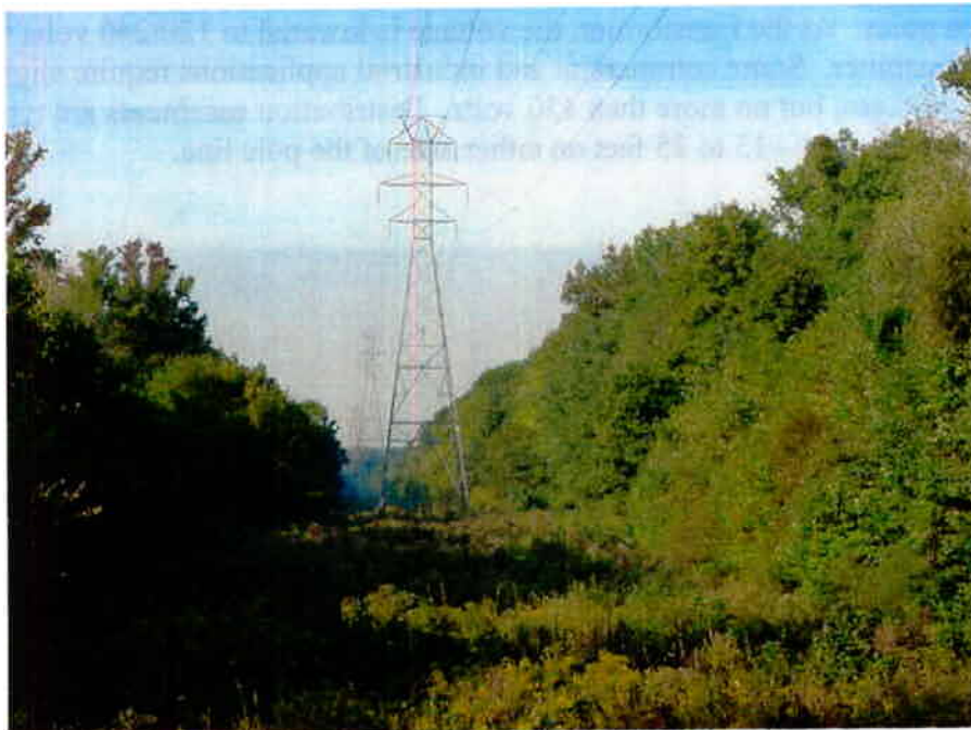
100,000 Volt Transmission Tower
